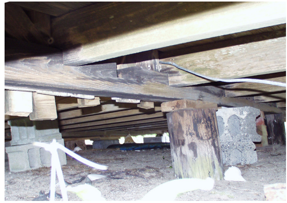
Figure 27 View of front sill of original house. Original siding extends below the bottom of the sill to left of center in this image. (NPS-SERO-CRS, 2002)
