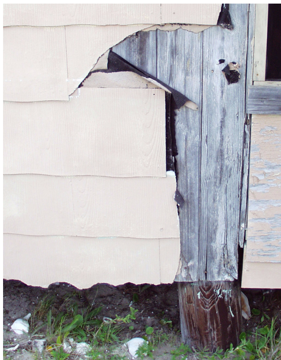
Figure 28 View of south corner of house showing original siding at center, asbestos siding at left, and modern plywood at right. (NPS-SERO-CRS, 2002)
