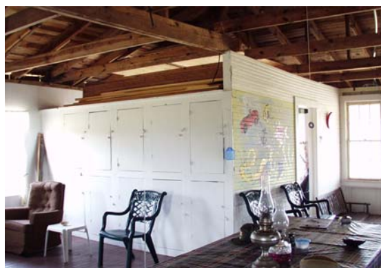
Figure 29 View west of built-in cabinets in southwest wing of cross hall. (NPS-SERO-CR, 2003)
