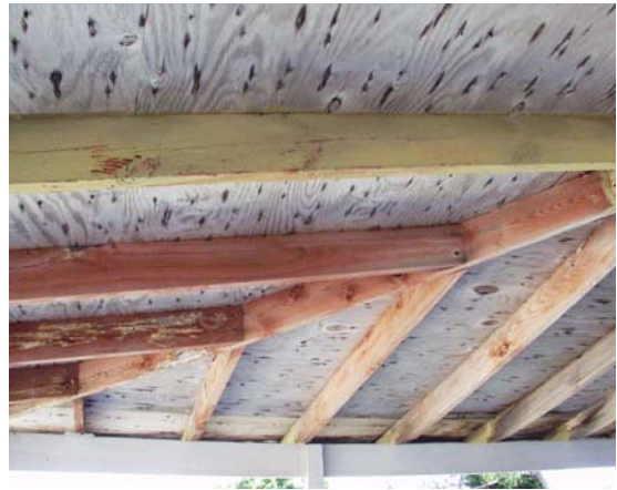
Figure 22 View of original porch roof framing at north corner of house. (NPS-SERO-CR, 2003)
