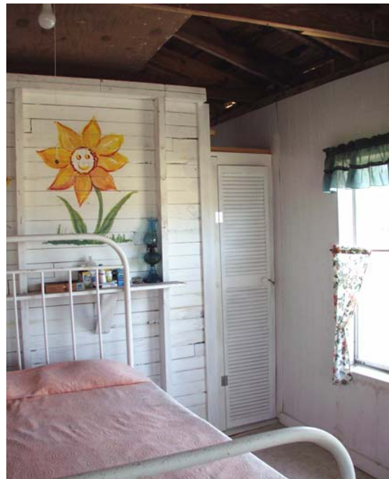
Figure 31 View south in Room 102, showing altered wall and added closet door. (NPS-SERO-CR, 2003)
