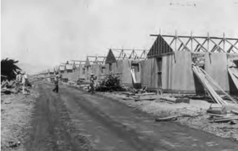
Buildings under construction at what will become the Poston War Relocation Center on the Colorado River Indian Reservation near Parker, Arizona, April 1942. The school complex in Unit 1 was designated a National Historic Landmark in 2012. Photo courtesy of the Library of Congress.
