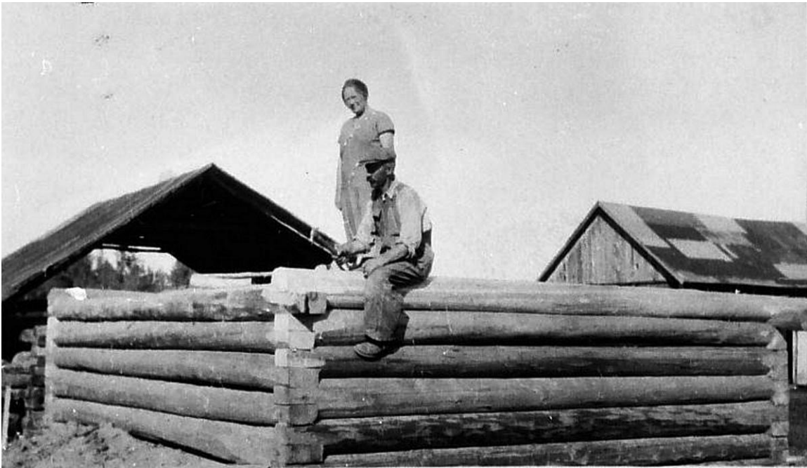
Figure 23. Bert and Birgit Noring building their root cellar, ca. 1913. Courtesy of Apostle Islands National Lakeshore, Noring Family Collection.
