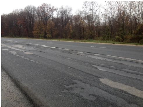
Road condition on the Baltimore Washington Parkway
