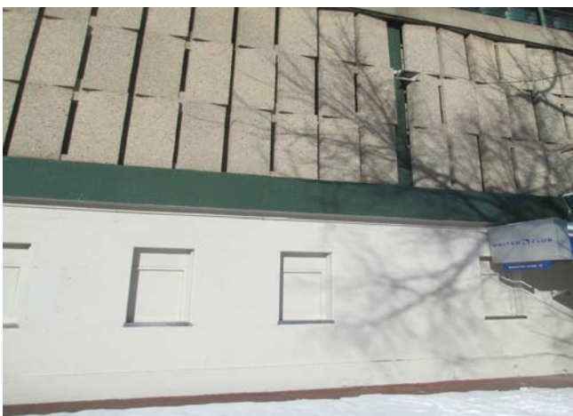
Possibly original stucco on the Addison Street elevation.
