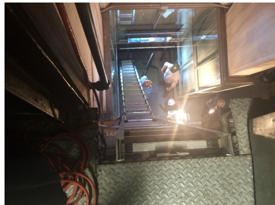
Figure 3: Observation Level Access to Machine Room Via Portable and Fixed Ladder
