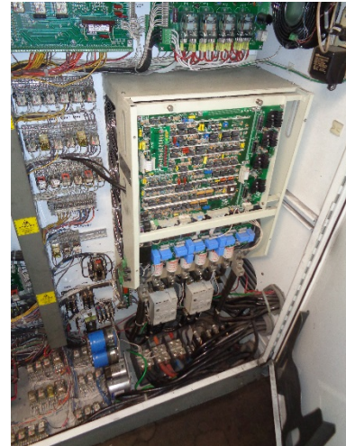
8. MCE controls need to be replaced.
