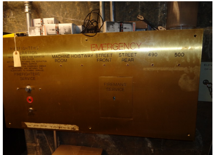
12. Existing fire control panel to be replaced.
