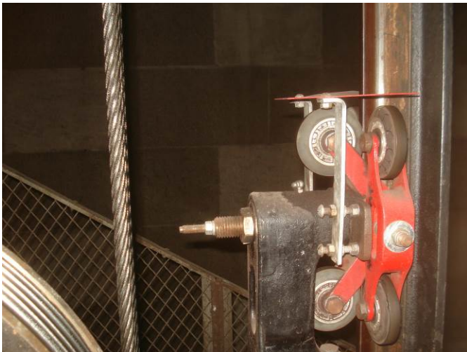
23. Chain link fence around hoistway is not safe or code compliant
