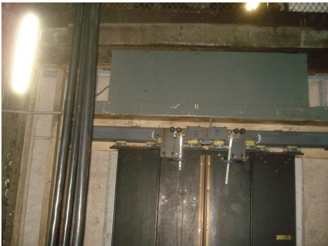
8. Replace missing dust covers
