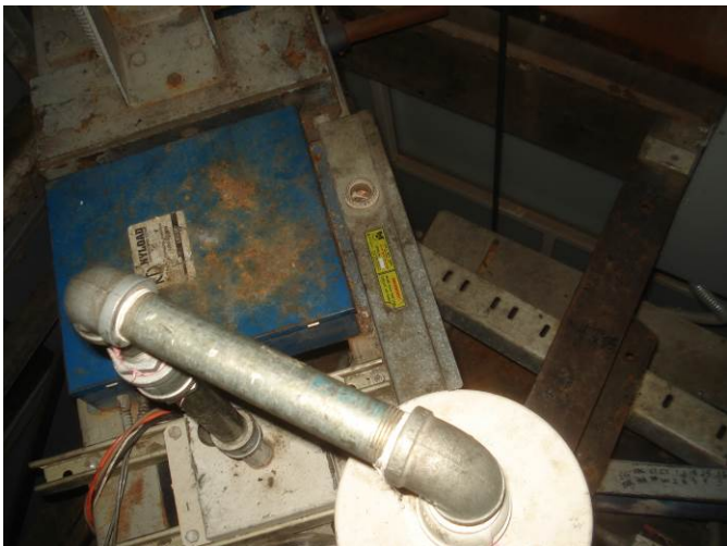
7. Cartop light needs to be operational
