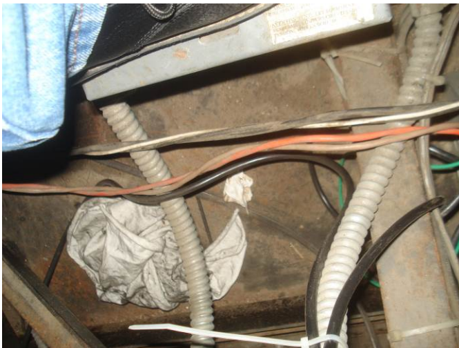
15. It is recommended that during the modernization, all CCTV wiring be placed in conduit.
