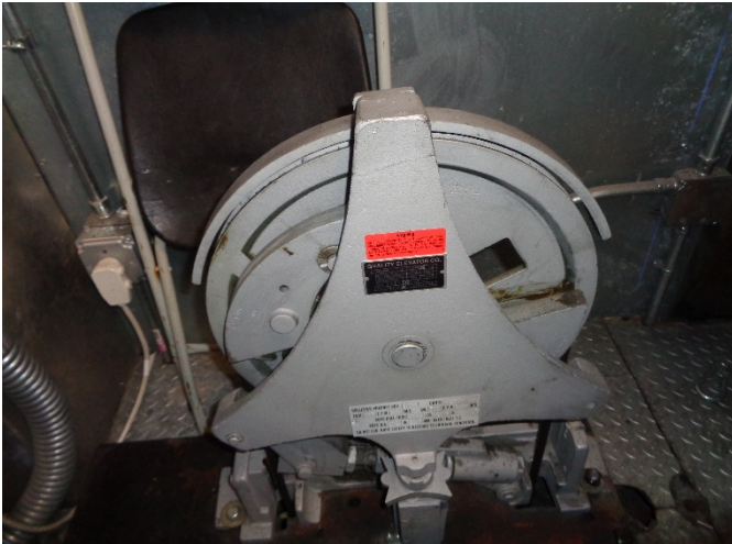
7. Dover Governor should be replaced.
