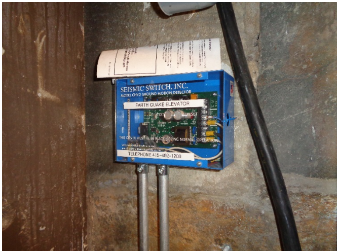
11. Existing seismic monitor to be retained.
