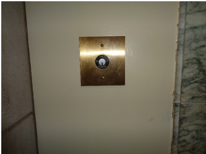
3. Existing wall mounted hoistway access switch
