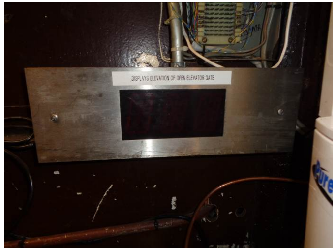
20. Repair position indicator in fire control room at ground floor
