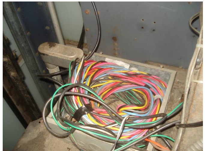
16. Replace missing electrical cover on junction box for CCTV camera at cartop
