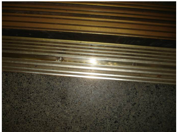
12. Car sill is worn and requires replacement
