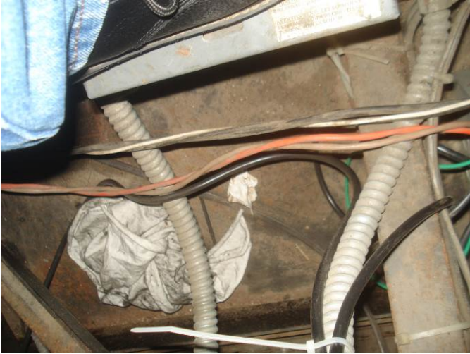
25. All wiring on car top should be protected.
