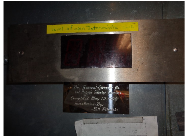
10. Existing car position indicator in machine room and security room does not operate. This will be replaced.
