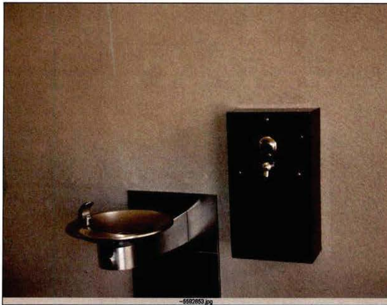
A newly installed water bottle filler at the Tucson Mountain District's Red Hills Visitor Center. Visitors were using the device before the installation crew had left the site!
