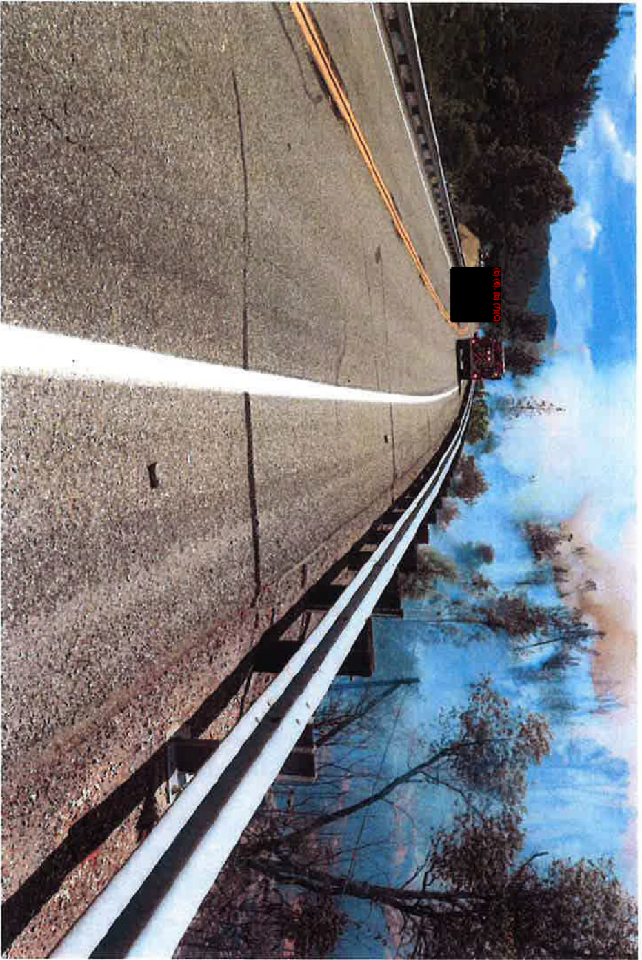
IMG_0009 Looking West with tire debris along Highway 299 West.
