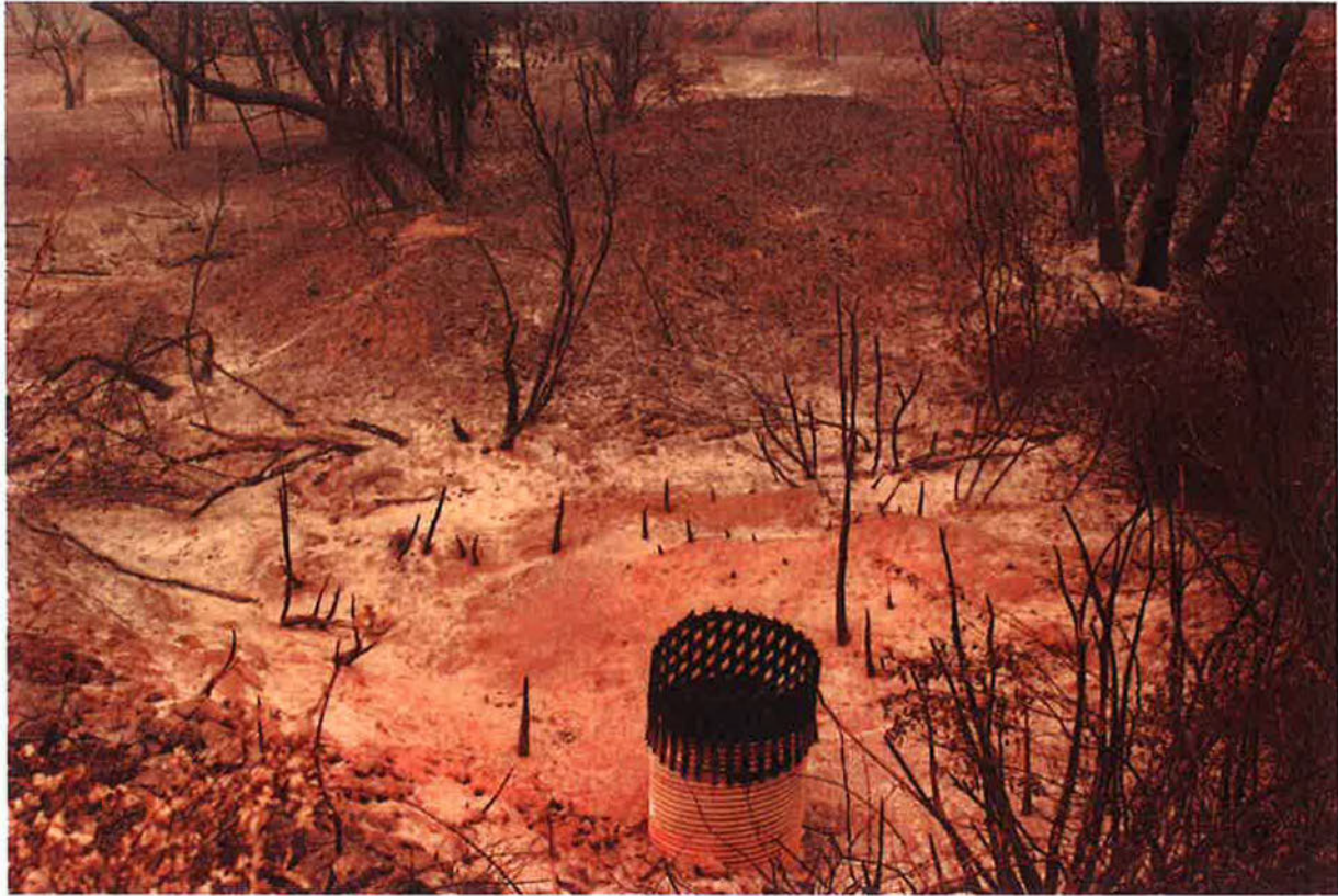
Photo 5 - IMG_0760 Fire B Drainage pipe at the bottom of the bowl area. This area was covered by green foliage on July 23, 2018.
