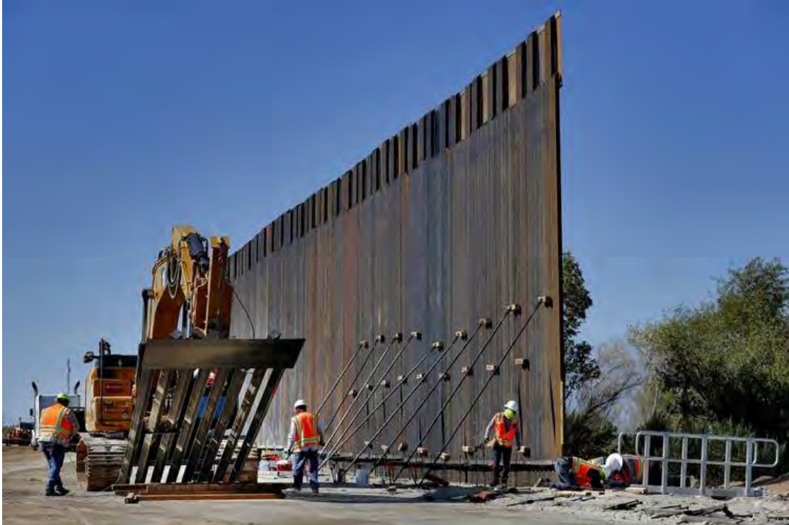
Government contractors erect a section of Pentagon-funded border wall along the Colorado River in Yuma, Ariz., in September. (Matt York/AP)
