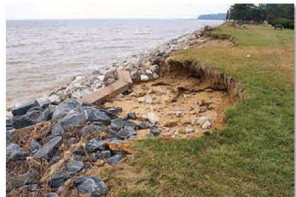
Shoreline erosion from storms.
