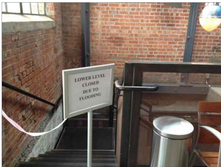
Photo 2. Basement flooding in the visitor center at Rosie the Riveter WWII Home Front National Historical Park. This photograph was taken on December 5, 2012 —12 years after the establishment of the park. Photo credit: Maria Caffrey.
