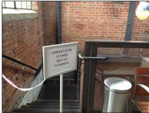
Photo 2. Basement flooding in the visitor center at Rosie the Riveter WWII Home Front National Historical Park. This photograph was taken approximately 12 years after the establishment of the park. Photo credit: Maria Caffrey.
