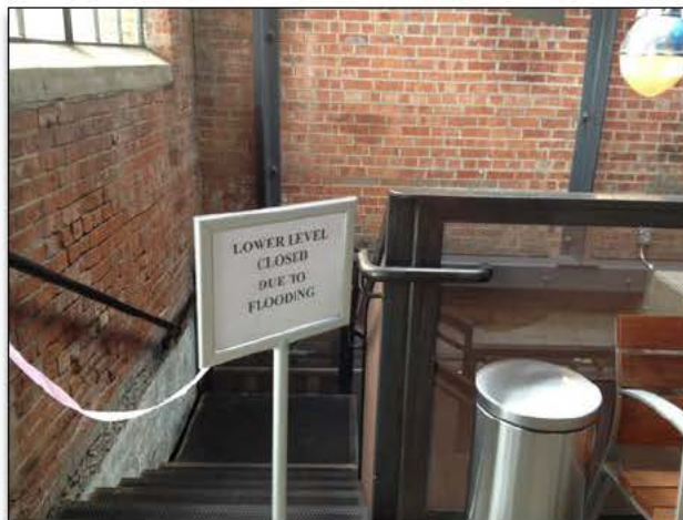
Photo 2. Basement flooding in the visitor center at Rosie the Riveter WWII Home Front National Historical Park. This photograph was taken approximately 12 years after the establishment of the park. Photo credit: Maria Caffrey.
