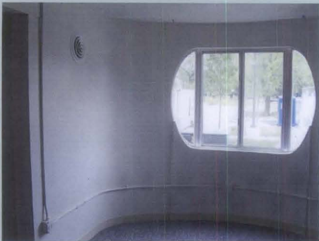
Figure e. Both interior and exterior aluminum surfaces had become dull, soiled, and oxidized as a result of traffic exhaust and air pollution. Cleaning the aluminum stabilized any further deterioration and brought back the luster of the original mill finish. (Photo: Holsten Real Estate Development Corp.)
