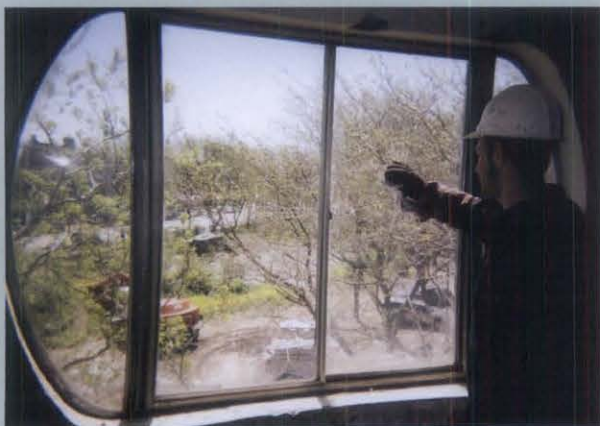
Figure f. Repair and replacement work was done from the inside to lessen the risk of damage to the outside finish. (Photo: Holsten Real Estate Development Corp.)
