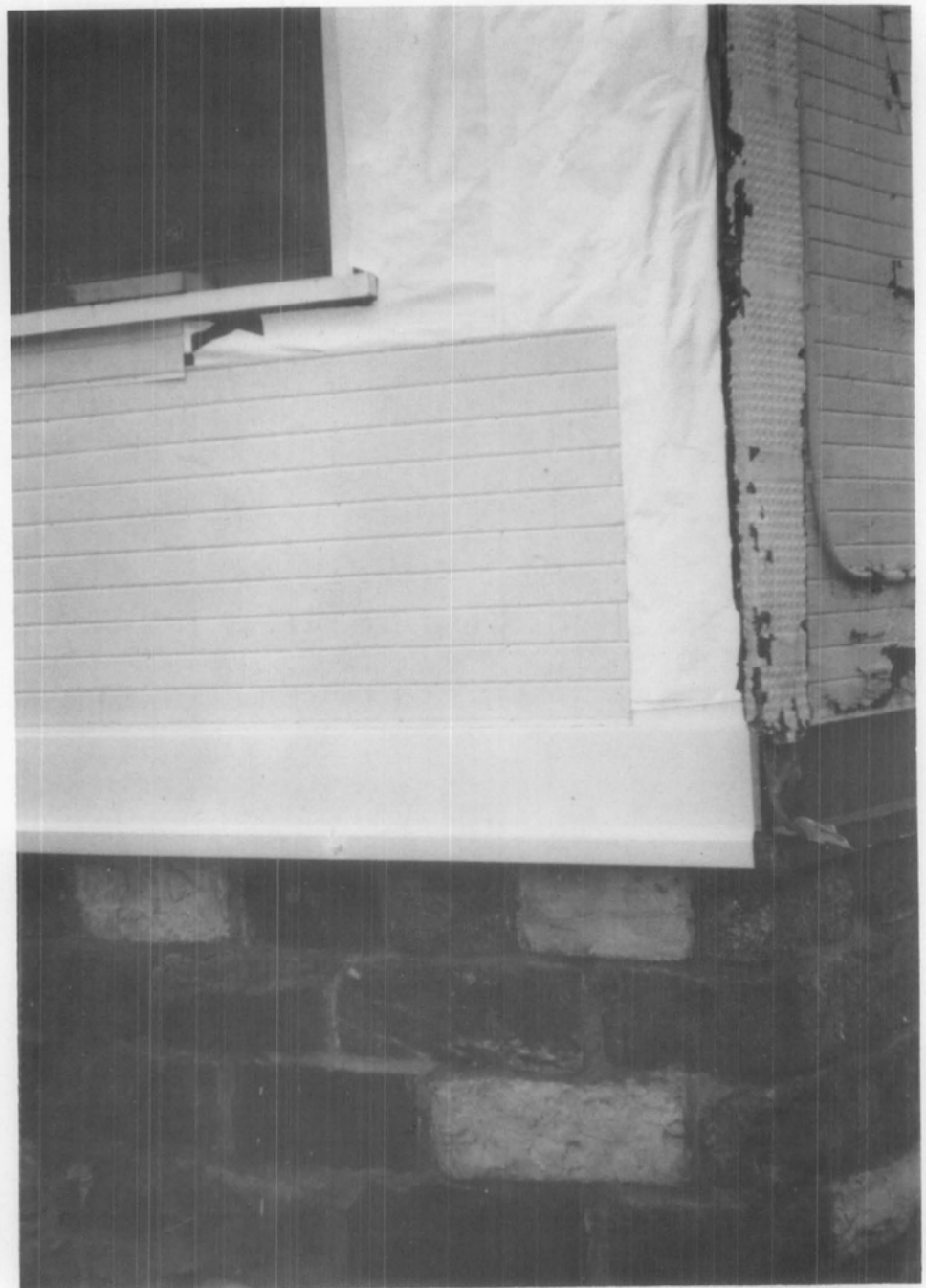
10. Installation of siding began at the base of each story of the building. Corner pieces were installed first, followed by the base flashing, and the stamped brick siding. Care was taken to match the patterns from one elevation to the next around the building. Photo: Mary Cay Bartush Jones.
