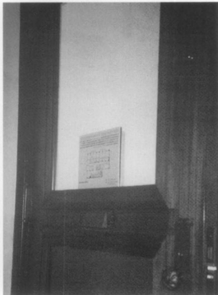
Figure 4. View of a Reliance Building office door from inside guest room. Upper and lower door panels have gypsum board secured to back with new molding. A mirror was affixed to the upper panel while the lower panel was painted to match original material. Photo: Chad Randl.
