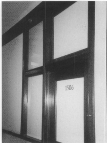
Figure 5. Completed Reliance Building corridor showing historic door panel, sidelight and transom. Photo: Chad Randl.
