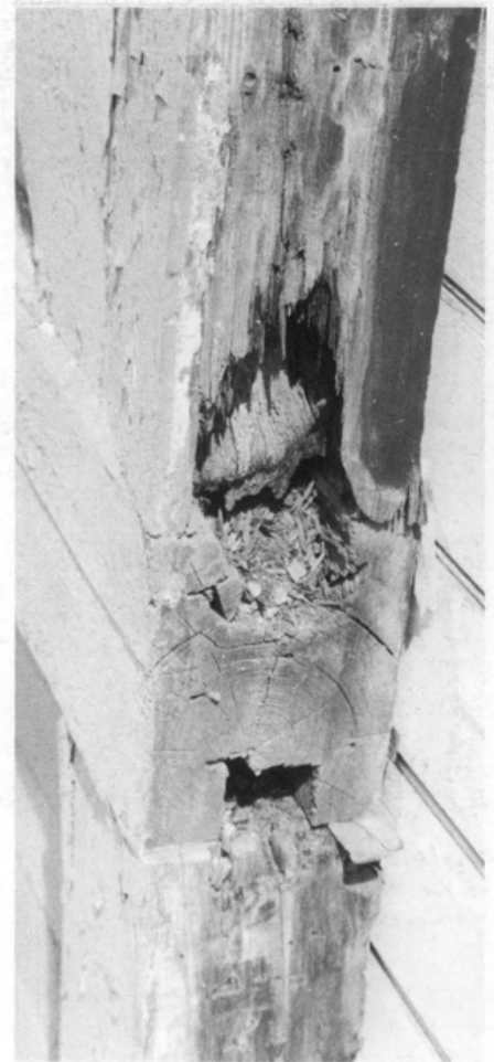
Figure 5. Some internal core deterioration was masked by sound surface wood. Water entering the connection of the post and beam framing rotted out the mortise and tenon pockets. These areas were consolidated and filled with epoxy. Photo: Baird Smith, AIA
