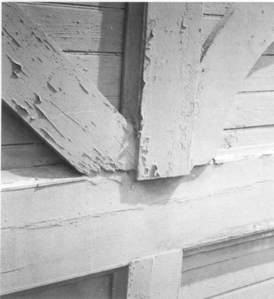
Figure 4. Flaking paint was the result of painting moisture-laden wood, using an inappropriate paint system, and undertaking the work during cold weather. Photo: Baird Smith, AIA
