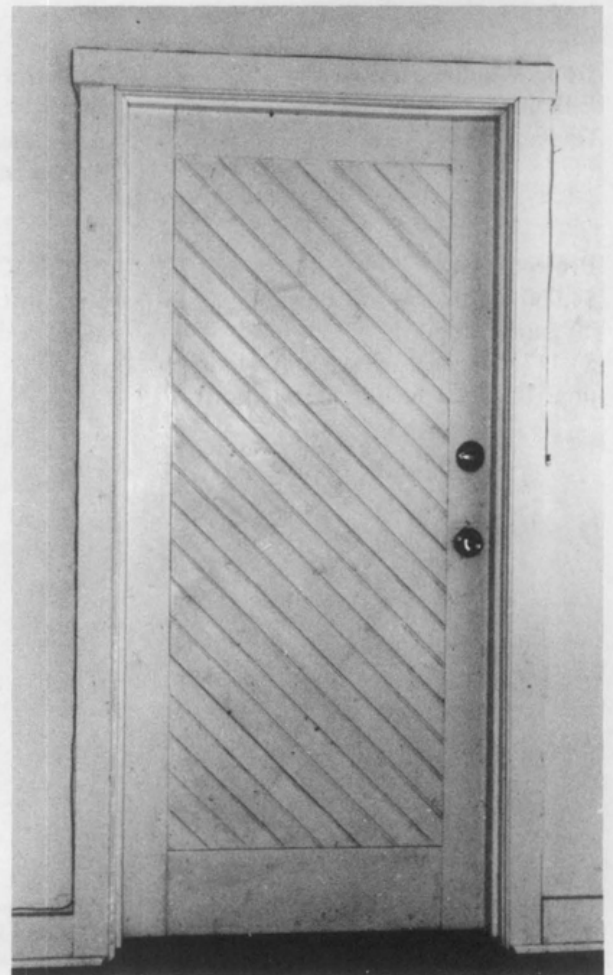
Figure 11. Diagonal boards used on the interior side of the door are in keeping with the utilitarian character of the building. Photo: Charles Fisher
