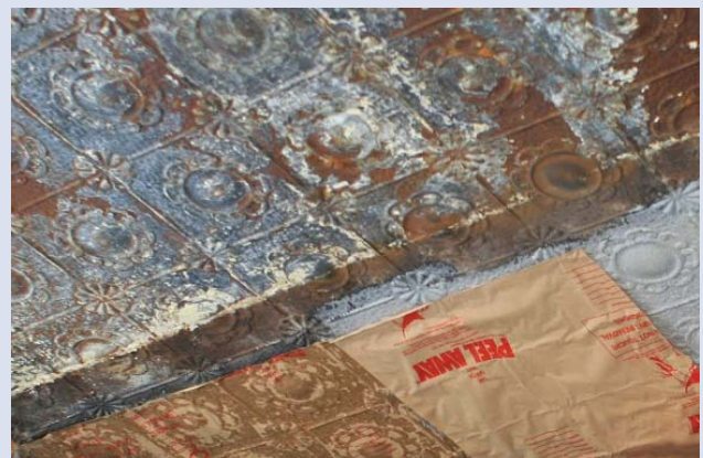
After applying a solvent-based paint to the metal, a laminated cloth/paper is applied during the chemical-peel process. (Photo: NPS)
