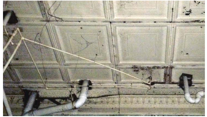
Metal ceilings can be greatly impacted by later penetrations from piping, electrical, and other such work, resulting in loose tiles and deflections in the ceiling. (Photo: Kaaren Staveteig, NPS)
