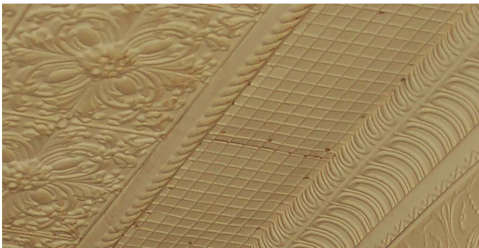
Some seams were easily disguised with interlocking patterns, whereas others, like butt joints, remained quite visible. Historic decorative metal ceiling at the LaSalle/Van Buren (CTA) station, Chicago, IL. (Photo: Kaaren Staveteig, NPS)
