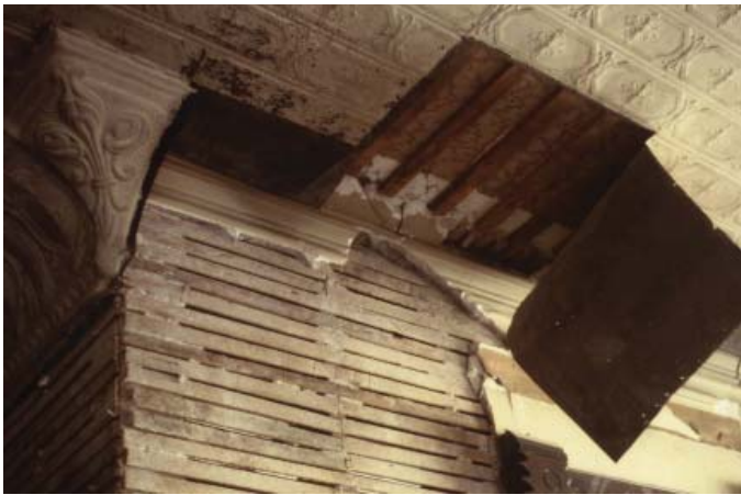
Prior to repair, a section of the pressed metal was removed to expose the condition of the plaster and lath and to document the earlier finish. (Photo: Kaaren Staveteig, NPS)
