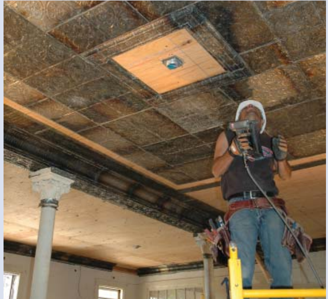
Figure d. Following the installation of the sound-proofing materials and drywall, the pressed-metal pieces were reinstalled using brads and a pneumatic gun. Matching the numbered pieces to the placement diagrams made the reinstallation easy.
