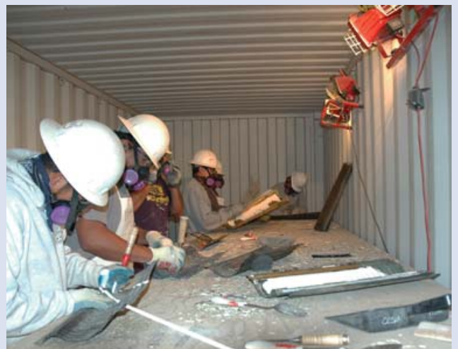
Figure b. On pieces where paint remained after the freezing/flex process, workers carefully hand-scraped with chisels to finish the clean-up. Because lead paint was present, workers were required to wear NIOSH approved-respirators.
