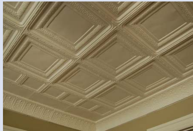
Figure e. The ceilings were finished with a fresh coat of paint. (Photos a-d courtesy of Kristin Baron, NPS; Photo e: Kaaren Staveteig, NPS)
