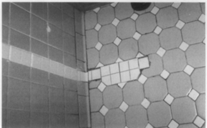
Figure 23. These non-matching tiles are inappropriate replacements for original tiles that were damaged during bathroom remodeling. Photo: Anne Grimmer.
