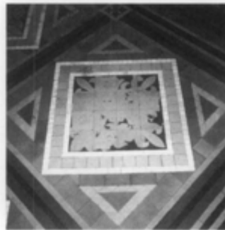
Figure 20. The surfaces of these late-19th century encaustic tiles have become worn and much of the pattern has been lost after more than 100 years of use. Photo: Anne Grimmer.
