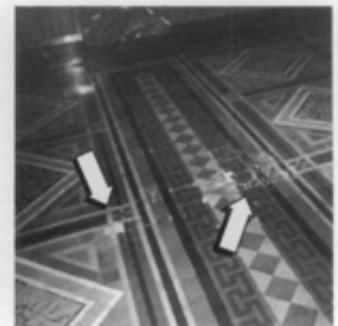
Figure 21. These cracked geometric tiles may have been damaged by the repeated passage of heavy equipment over the floor. Photo: Anne Grimmer.
