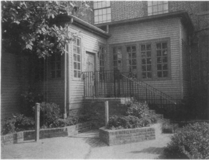
Figure 14. At the Lieutenant Governor's Mansion in Frankfort, Kentucky, a retracting lift (b) was installed to minimize the visual effect on this historic building when not in use (a). Photos: Aging Technology Incorporated.
