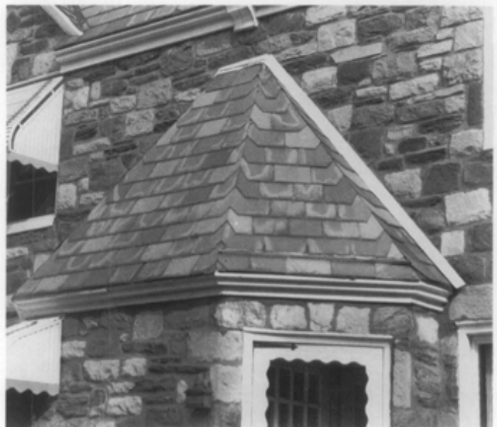
Figure 14. The white blotches on these Pennsylvania Soft-Vein slates indicate areas where gypsum is leaching out onto the surface of the slates.
