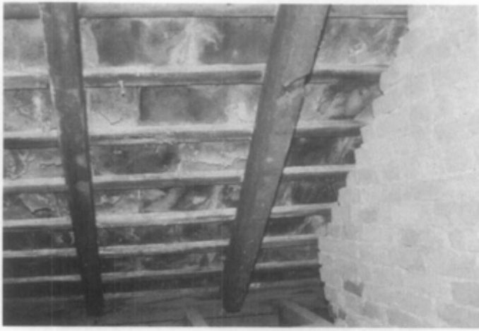
Figure 15. View of the underside of slates laid on open sheathing shows that delamination and flaking is just as bad or worse on the underside of slates as on the exposed surface. This is why most slates cannot be flipped over for reuse.
