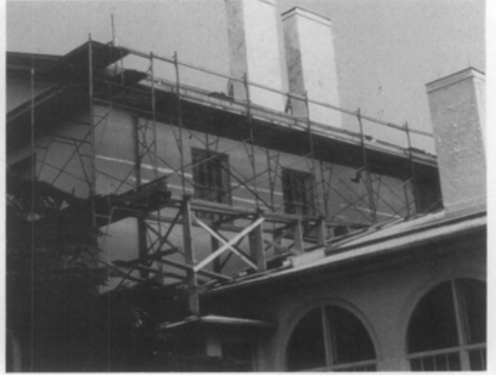
(b) Scaffolding was installed early to document existing conditions to determine extent of work.
