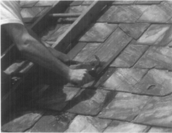
(a) A ripper is used to remove the nails from the deteriorated slate.
