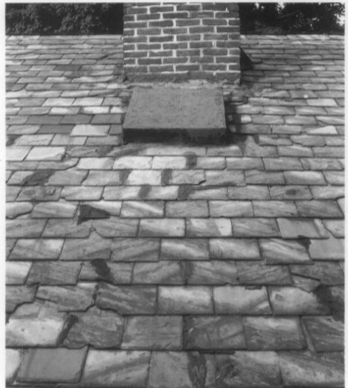
Figure 20. This roof has been poorly repaired numerous times in the past. The installation of mastic to seal out moisture has only exacerbated the problem. A timely repair and good maintenance could have extended the life of this roof.
