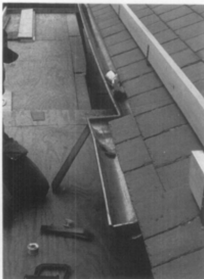
(i) Although the gutters and snow boards were the last elements installed, their support brackets were installed as the slates were laid.
