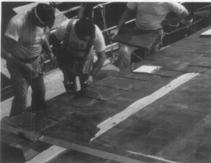
(e) Roofing felt was installed over decking; a rubberized membrane was used selectively at the eaves and under some flashing.
