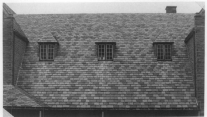
Figure 5. This graduated slate roof is composed of large, thick slates at the eave which are reduced in size and thickness as the slating progresses to the ridge.
