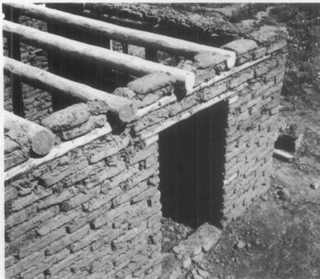
Roof Bearing. A roof bearing timber placed within the adobe walls provides even support for the weight of the roof. (Farm Security Administration Collection, Library of Congress)
