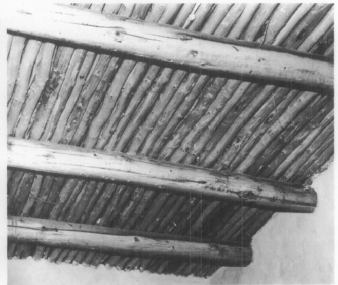
Roof Framing. Viga logs and savinos are seen in the interior of the adobe building. Often the wooden materials that compose the traditional flat adobe roof create interesting and pleasing patterns on the ceilings of the interior rooms. (Photo by Russell Lee, Farm Security Administration Collection, Library of Congress)
