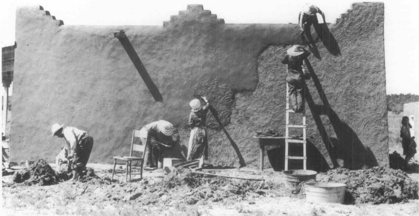
Renewing the Surface Coating. Traditionally, adobe surface coatings that protected the fragile adobe building fabric were renewed every few years. Recently however, high labor costs have made this a relatively expensive process. Women are seen here recoating an adobe wall with mud plaster mixed with straw at Chamisal, New Mexico. (Photo by Russell Lee, Farm Security Administration Collection, Library of Congress)
