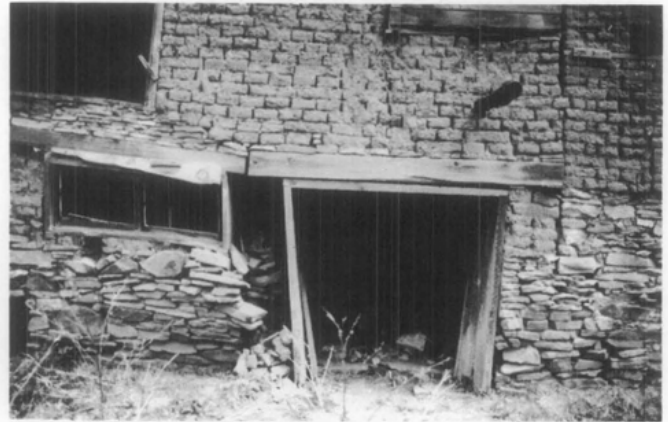
Structural Damage and Cracking. Sagging, bulging, and cracking of walls and roofs are signs of serious problems in the adobe building. It is always advisable to secure professional services in the repair of such problems. (National Park Service)
