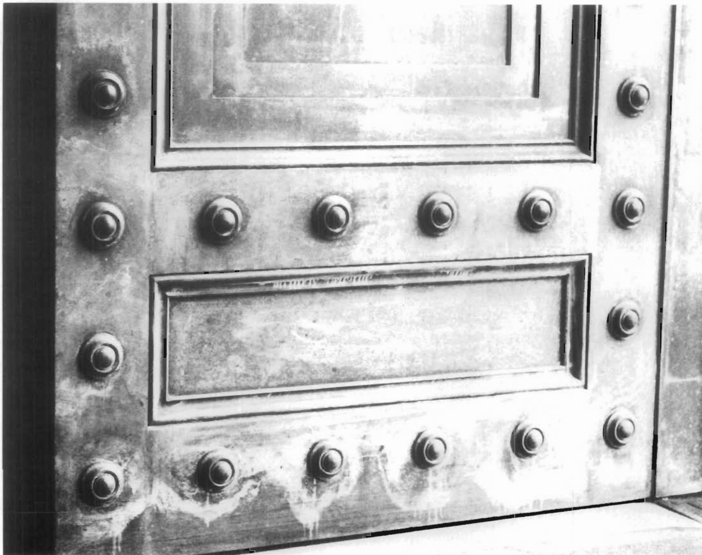
Figure 153. Improper Cleaning of Bronze. The bronze doors on the Pennsylvania Avenue side of the National Archives in Washington, D.C., were cleaned improperly. They now vary in color from a golden bronze to green to copper orange and brassy yellow. Some of the original artificial patina applied at the foundry has been removed, leaving a blotchy appearance. Part of the corrosion from the deicing salt remains, and the doors have a streaked, unattractive appearance. At this point, the only feasible treatment would be to clean the doors thoroughly (down to the bright metal), by mild chemicals or soft abrasive cleaning. A new artificial patina could be applied to return the doors to their original appearance. To protect against future damage, the doors should be given a barrier coating of wax which will need to be renewed periodically. The maintenance staff should be notified not to use salt near the doors and not to clean or polish the doors other than washing them down once a year with a nonionic detergent. When washed, the doors should be thoroughly rinsed with distilled water and wiped dry with a clean cloth to prevent water spots and streaks. (David W. Look)
