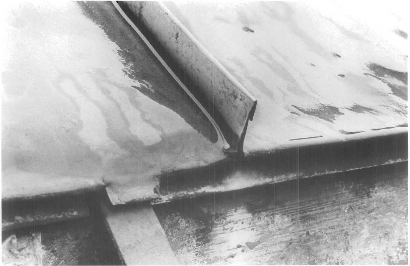
Figure 150. Erosion of Copper. This eaves detail of the 1920s copper roof on the Senate House State Historic Site in Kingston, New York, illustrates erosion of the copper at the edge of the roof caused by continued exposure to rain and snow, which scoured the roof as it flowed to the gutter. Fatigue failure has also occurred at the base of the standing seam, resulting in a tearing of the copper. This failure was caused by the lack of provision for expansion and contraction, as well as the use of bituminous roofing felts, which restricted the movement of the copper. (John G. Waite)
