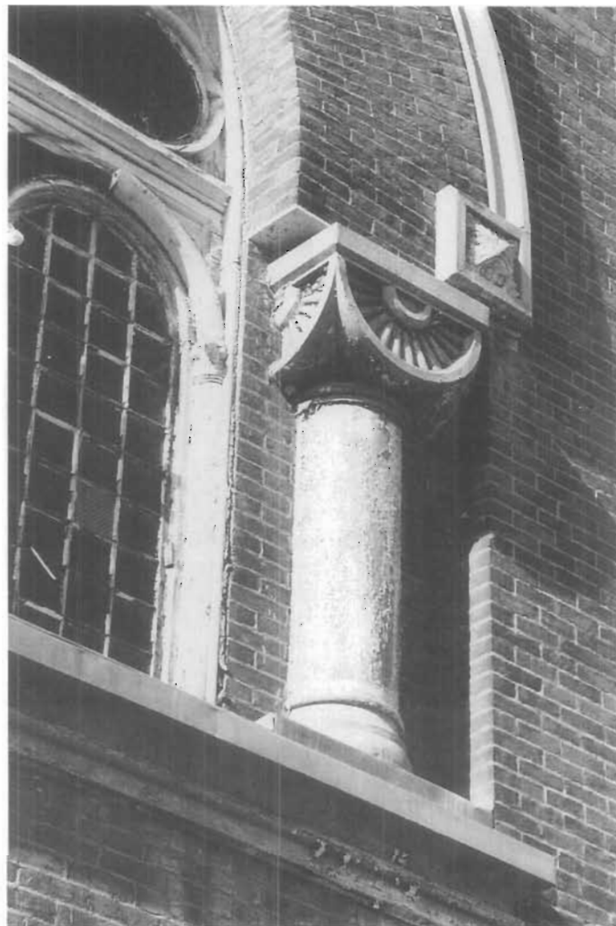
Figure 138. Zinc Deterioration and Staining. On the First Presbyterian Church in Alexandria, Virginia, the engaged columns, arch molding, corner blocks, and the sill molding are fabricated of cast zinc and galvanized sheet iron (the windows and frames are wood). The paint has deteriorated, leaving the surface of the metal bare in some places. The zinc or zinc coating on iron has oxidized. Notice the whitish corrosion stain on the brick from the zinc carbonate coating which continues to wash over the surface of the bare metal and then down over the bricks. The metalwork should be scraped down to remove all loose zinc carbonate. Joints should be caulked and/or resoldered, and repainted with a zinc chromate primer. (Baird M. Smith)
