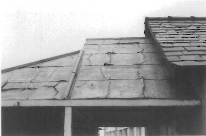
Figure 119. Creep. Deterioration of milled sheet lead roof on a 19th century canal warehouse and office at Nantwich Basin of the Shropshire Union Canal at Nantwich, Cheshire, England. The failure has been caused by creep and the expansion and contraction of the lead. (John G. Waite)
