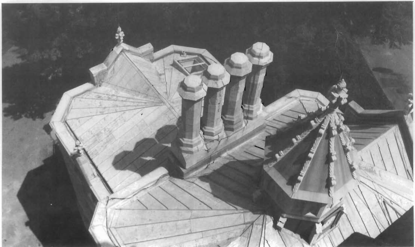
Figure 135. Complete Substitution of Lead-Coated Copper Roofing for Terneplate Roofing. The 1864 wing addition of Lyndhurst, Tarrytown, New York, originally had a terneplate roof. In an attempt to find a more permanent roofing material, a lead-coated copper roof was substituted for the terneplate, duplicating the pattern and sheet sizes of the original roof. In such substitutions, details may have to be redesigned because of differences in expansion and contraction rates and differences in workability of the material. The color of lead-coated copper is not the same as terneplate because terneplate roofing was never left unpainted. Therefore, lead-coated copper roofing substituted for terneplate should also be painted if it seen from normal viewing angles (usually from street level). (John G. Waite)
