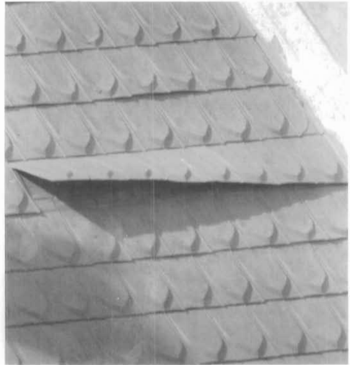
Figure 123. Anchorage Failure. The nails holding down this section of embossed galvanized sheet-iron roofing have deteriorated and the wind has lifted up the corner of the sheet, allowing water to leak through the roof sheathing. Other sections (not shown in the photo) had flapped in the wind until the sheet metal cracked with fatigue failure and tore loose. In 1977 this roof at St. Edward's University in Austin, Texas, was cleaned and supplemented with reproduction "shingles" where needed. (St. Edward's University)
