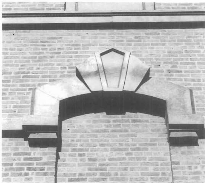
Figure 137. Deterioration of Zinc. At the 1874 Cohoes Music Hall, Cohoes, New York, the original zinc window lintels and belt course were cleaned by sandblasting, resulting in pitting and corrosion of the metallic surface. Note the whitish corrosion products caused by the abrasive cleaning and subsequent exposure to the weather. The lintels had been painted originally but were left bare after the cleaning. Zinc and galvanized sheet iron should always be primed and painted with paints especially formulated for zinc. (John G. Waite)
