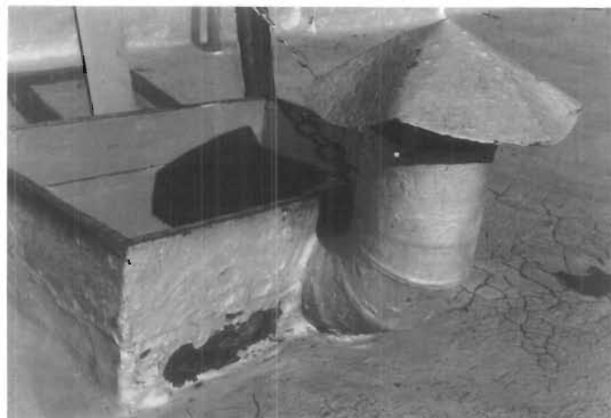
Figure 128. Deterioration of Tinplate by Asphalt Coating. The tinplate flashing of the roof hatch has been corroded away (between the corner and the vent) by the action of the asphalt coating and water. (John G. Waite)
