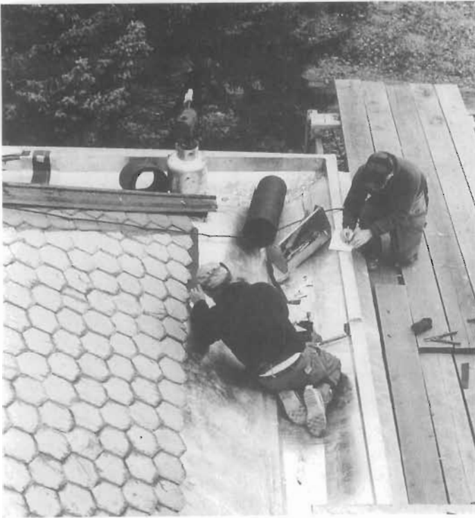
Figure 134. Replacing Flashing and Gutters. Workmen replaced the deteriorated terneplate flashing and gutters at Olana, built between 1870 and 1874 near Hudson, New York, for the noted artist Frederic E. Church. The polychromed slate roof was restored to the original pattern, and lead-coated copper was substituted for the original terneplate flashing and gutters because of ease of maintenance - it does not require painting, unless there is a need to match the terneplate in color. The original terneplate was painted. (John G. Waite)
