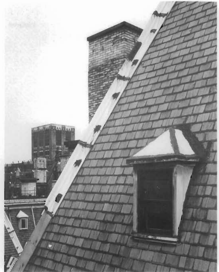
Figure 148. Inappropriate Patching Compounds. Corrosion of a copper roof ridge on the Dakota Apartments (1884), New York City, was caused by the use of an asphalt roofing compound for temporary patches over nailheads and joints between ridge sections. (John G. Waite)
