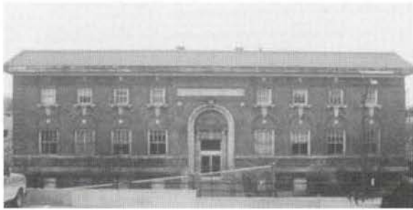
The Sioux City Free Public Library prior to rehabilitation. The building had major structural problems after sitting vacant for over ten years.
