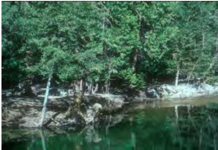
Figure 1: Left bank at Housekeeping Camp. Exposed roots in the foreground; riprap boulders in the background.
