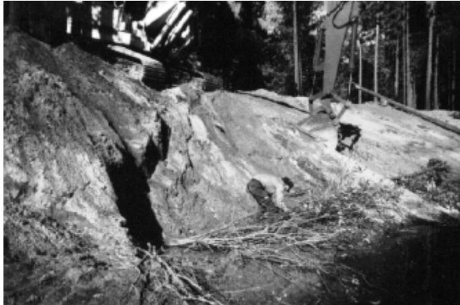
Figure 1: Crew member planting willow and cottonwood cuttings with the aid of the excavator
