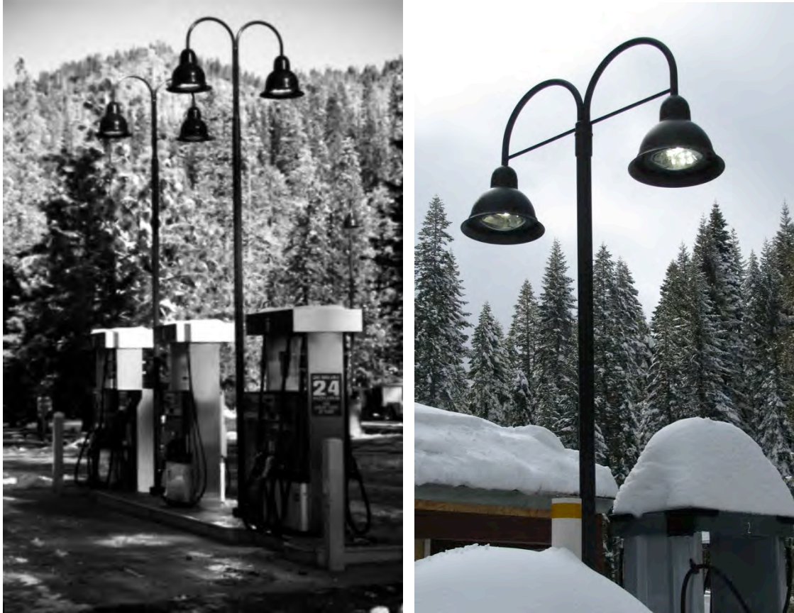
Figure 5 –Tall Pole Lights at (l.) Wawona Gas Station (r.) Crane Flat Gas Station. This design was developed prior to the completion of these Guidelines. Fewer lumens (lower wattage lamps) should be used on similar installations in the future.
