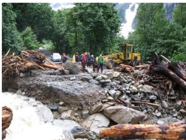
Figure 14. Cascade River Road, August 2013. Heavy rain mobilized river debris clogging a culvert. The road washed out, stranding 70 visitors and their vehicles for 2 days. (Source: NPS)
