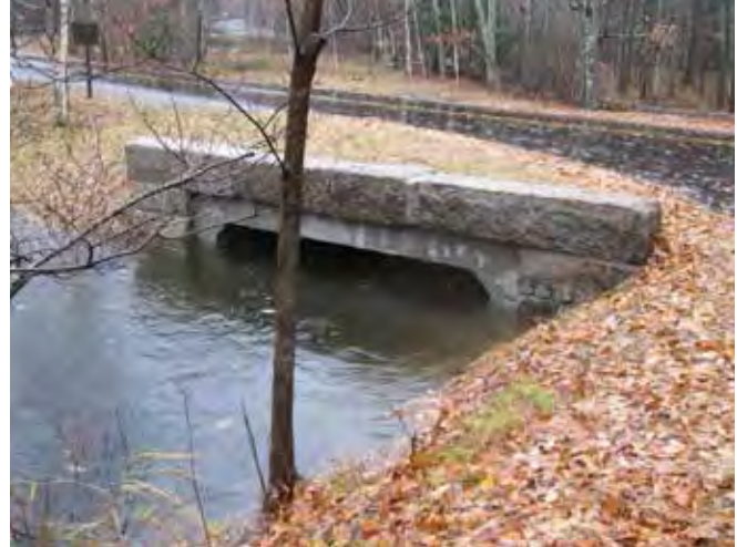
Headwall and culvert after rehabilitation at Sieur de Monts Spring site. Image credit: Rebecca Cole-Will.
