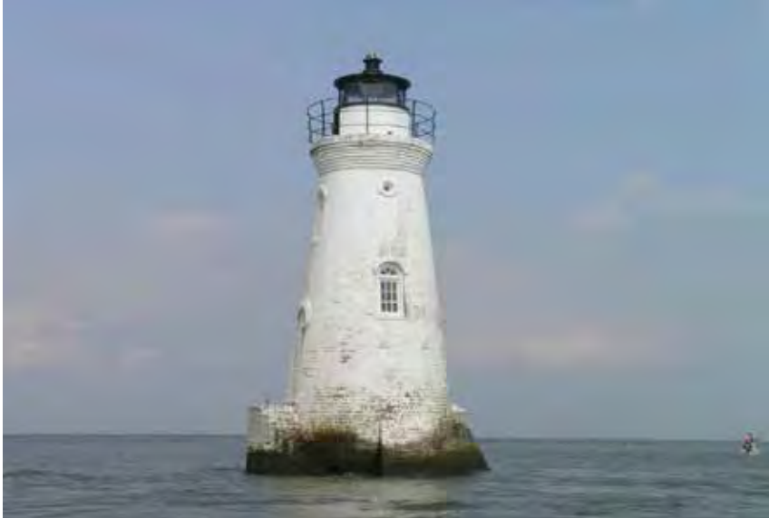
The Cockspur Lighthouse at Fort Pulaski National Monument needs to be stabilized. Image credit: Mike Eissenberg, NPS.
