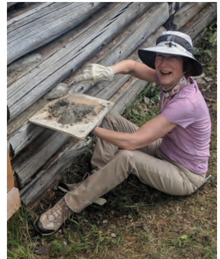
Daubing seals the space between the logs making the structure weather tight.
