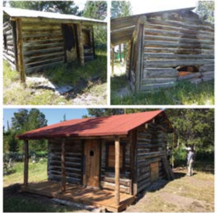
A Bar BC cabin shown before and after the Grand Teton Hammer Corps volunteers repaired and stabilized the structure.
