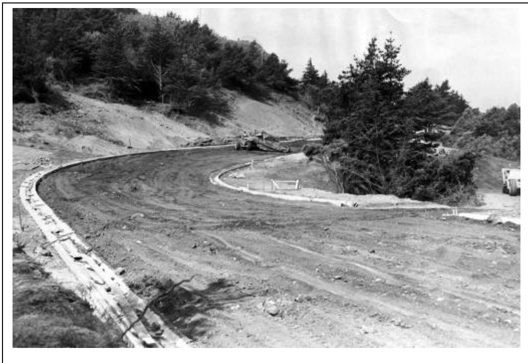
Figure 73. Reconstruction work on El Camino Del Mar below Fort Miley, May 17, 1951. New drainage swales are visible along both sides of the graded roadbed. (SF Public Library AAB-3499)
