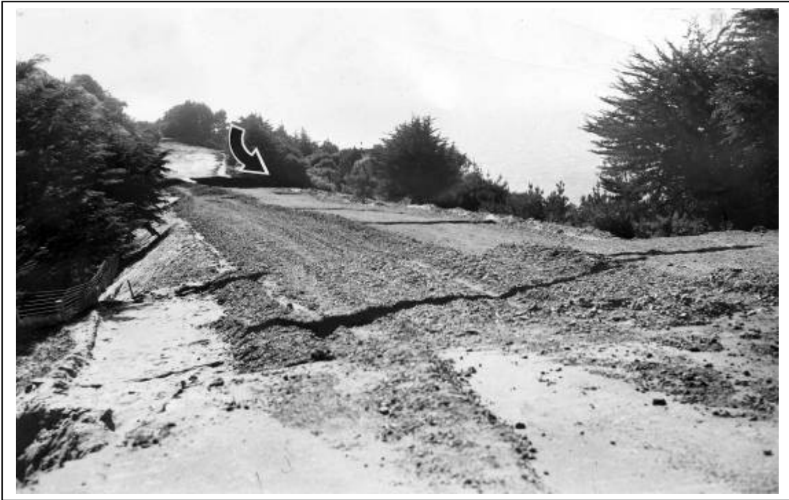
Figure 76. Arrow indicating a slide on El Camino Del Mar below Fort Miley, 1941. View west. (SF Public Library AAB-9153)
