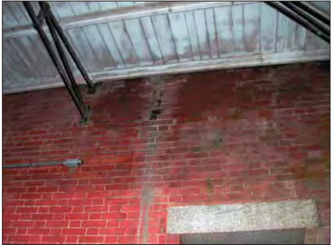
Condition Photo 12: Southwest Courtyard Elevation— Third Tier by Stair 1; Roofing materials are saturated from improper drainage at the barbette tier. The wood appears to be deteriorated. Biological growth has settled on the roofing materials and the masonry. Paint coatings are no longer extant. (Courtesy of ARG, 2003)
