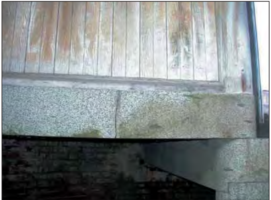
Condition Photo 6: Top Landing at Barbette Tier; Crack in granite. (Courtesy of ARG, 2003)
