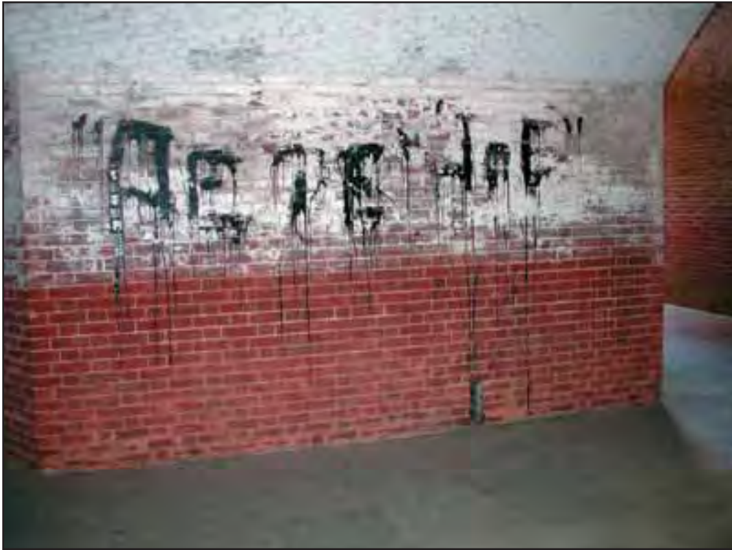
Condition Photo 18: Casemate 68A—Second Tier; Graffiti noted on masonry wall. (Courtesy of ARG, 2003)
