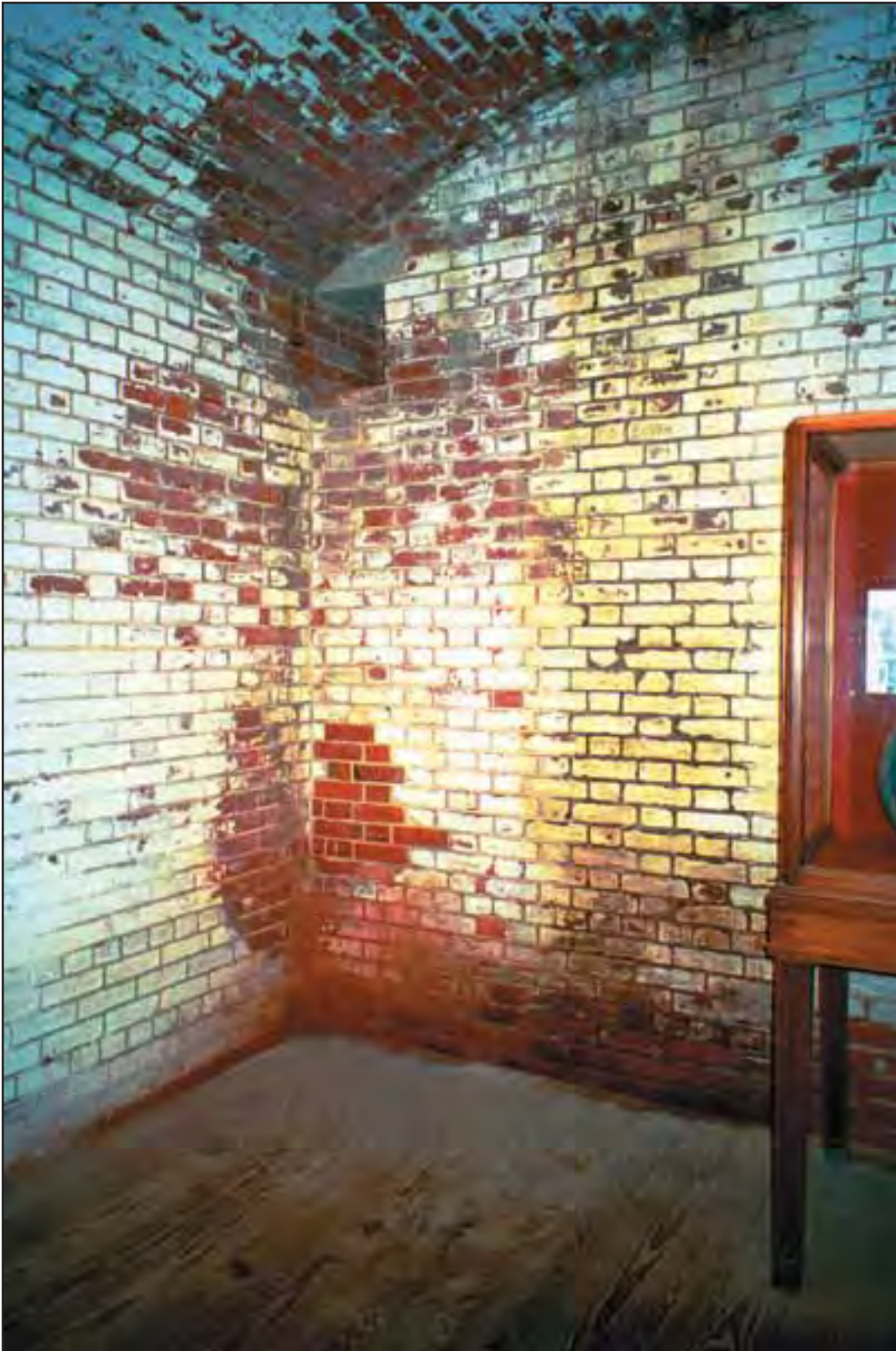
Condition Photo 16: Casmate 11; Open joints at the brick masonry and heavy water infiltration. Biological growth on the interior brick. (Courtesy of ARG, 2003).
