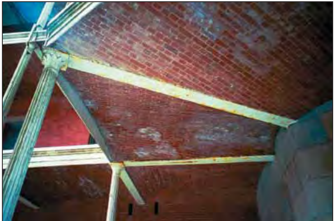
Condition Photo 9: Southeast Courtyard—Underside of Walkway at Tier One; Metal corrosion and staining of the granite walls. The brick facing is spalling. Efflorescence occurs on the brick and granite masonry. (Courtesy of ARG, 2003)
