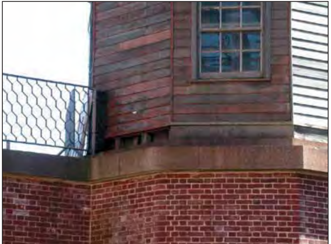
Condition Photo 13: Stair 3; Missing siding exposes the structural framing. (Courtesy of ARG, 2003)
