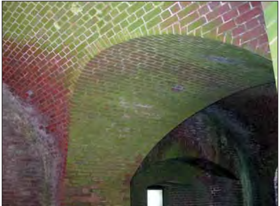
Condition Photo 2: Intersecting Arch of Casements 98 and 99; Biological growth and efflorescence settle on masonry surfaces. (Courtesy of ARG, 2003)
