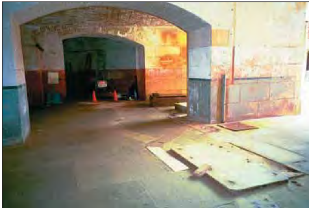
Condition Photo 19: Casemate 34; Uneven surfaces, open holes and potential tripping hazards. (Courtesy of ARG, 2003)
