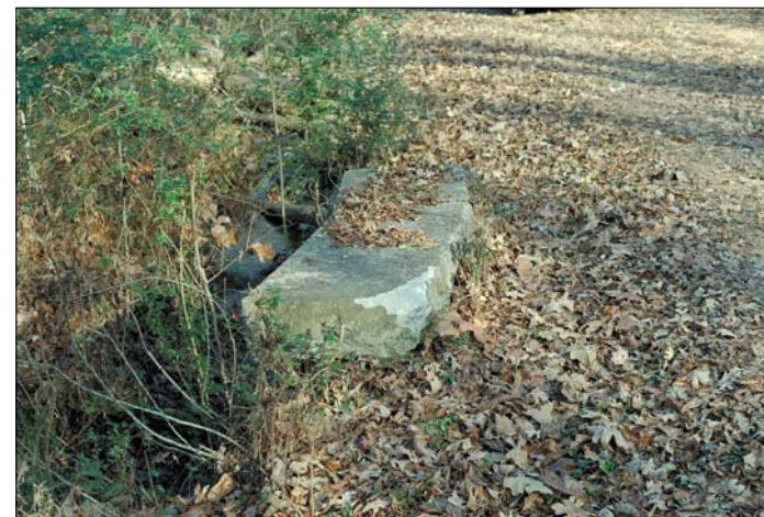
Example of headwall along Mullis-Vittetoe Road that has been damaged by road equipment and overgrown with vegetation.
