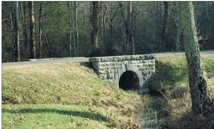
Existing conditions photo of same culvert. Original drawings should become an element of the preservation maintenance plan.
