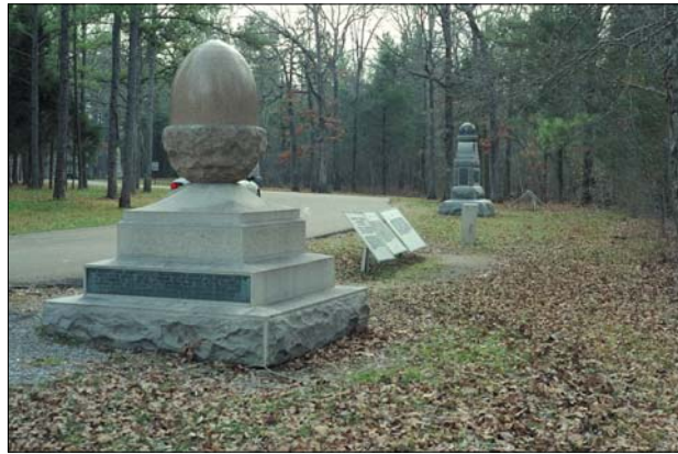
Engraved text on some of the monuments has become difficult to read over time. These inscriptions should be documented, and cleaned in consultation with a materials conservation specialist.
