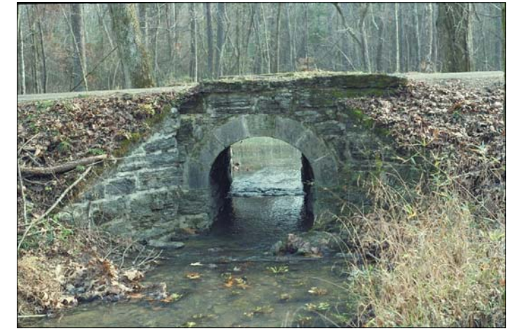
Example arch culvert. Location, condition, materials, and construction and maintenance records information should be collected for each culvert within the Park.
