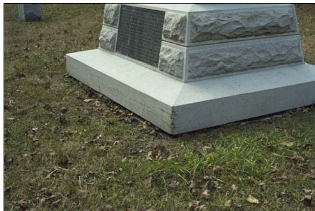
Example of damage resulting from lawn mower blades. Educate maintenance employees to ensure no further damage to monuments occurs due to maintenance practices.
