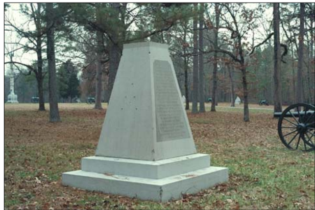
Some monuments and markers have components missing. This should be documented in the condition assessment.
